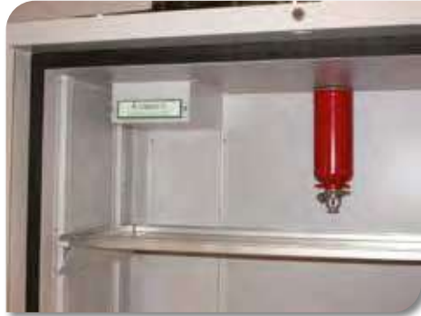
Fire-extinguisher installed in a safety cabinet
